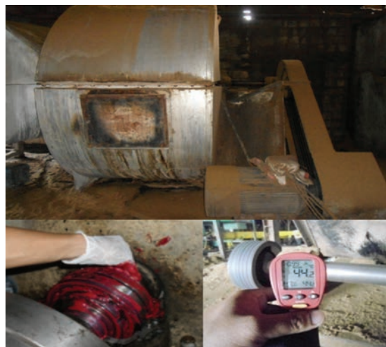
Induced Draft Fan of Boiler and Fiber Blower Units
